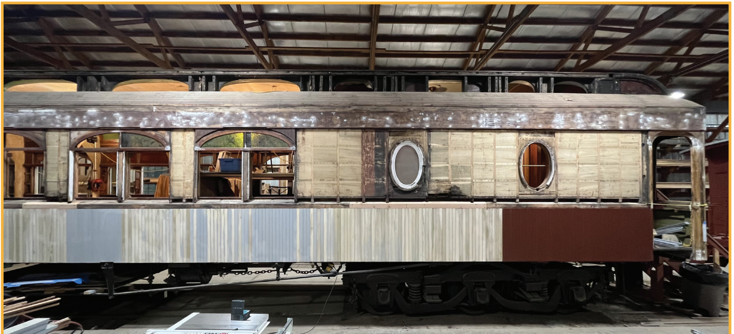
Some of the new lower siding installed on the car. The portion on the right has the first coat of Tuscan Red tinted primer.
