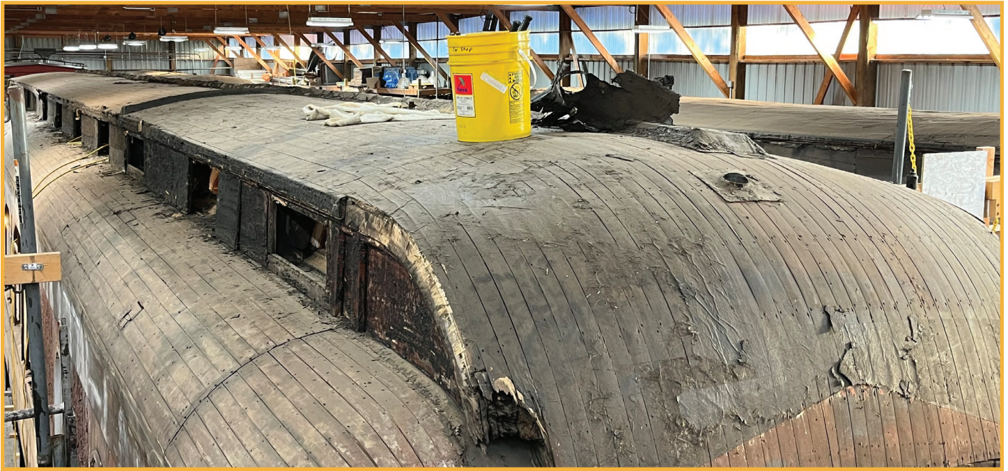
Before the upper roof wiring, wire trough, and metal enclosure were dismantled and removed.
